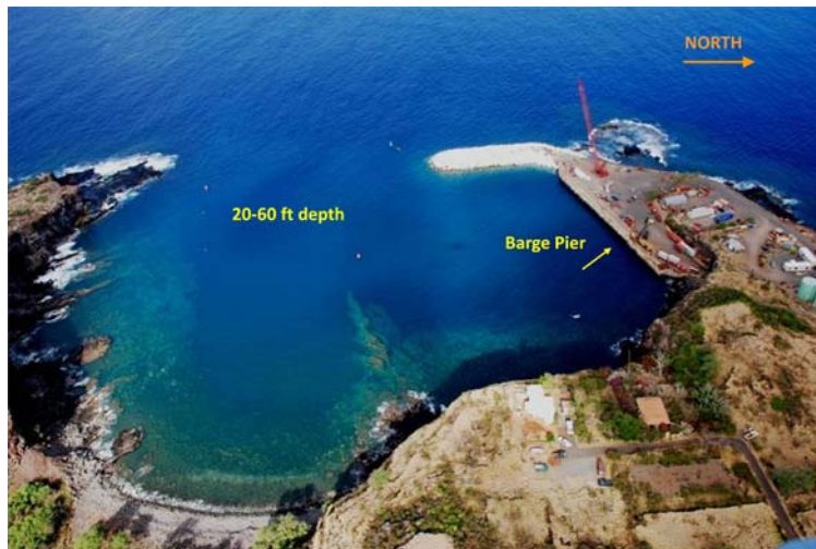
Figure 2. Breakwater under Repair at Kaumalapau Harbor.
